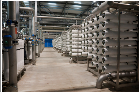
RO (Demi Water Plant, Botlek)
