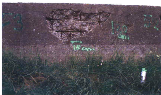
Plate 3: Viane, Dijkpaal No. 333 + c.54m: Large area of spalling in wall. Reinforcement visible. Approximate dimensions marked on wall.
