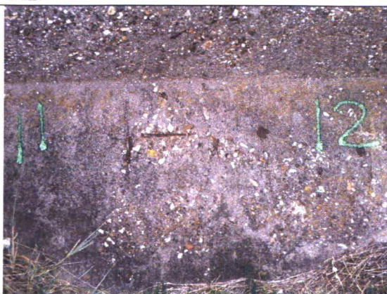
Plate 5: Schelphoek, Dijkpaal No. 55 - c.67m: Reinforcement visible on concrete slope.
