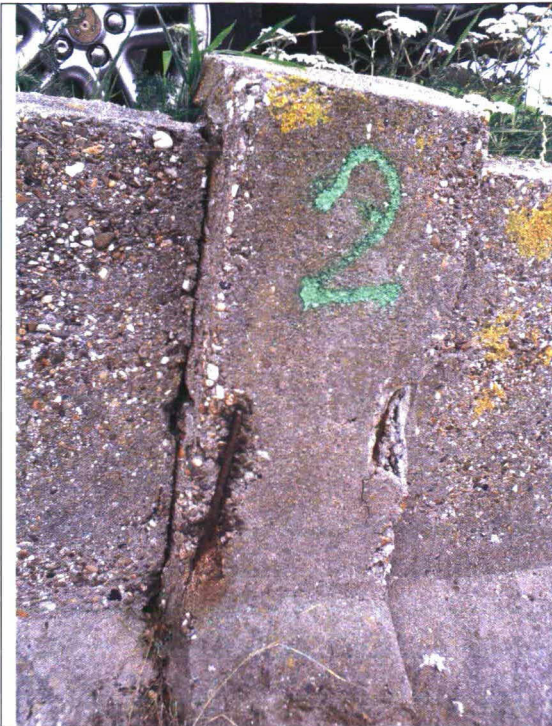
Plate 7: Schelphoek, Dijkpaal No. 55 – c.90m: Reinforcement visible on post.
