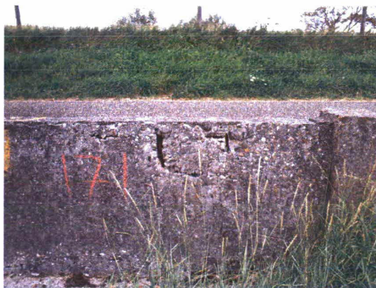
Plate 1: Viane, Dijkpaal No. 329 + c.63m: Spalling evident in wall. Reinforcement bars visible.
