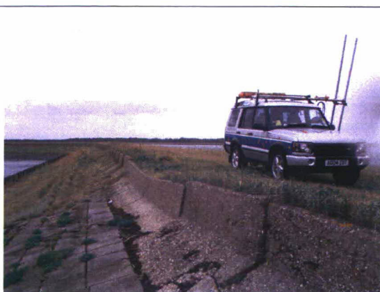
Plate 6: Schelphoek, Dijkpaal No. 55 +c.1327m Change in construction at end of dyke (near survey limit) at Schelphoek West.
