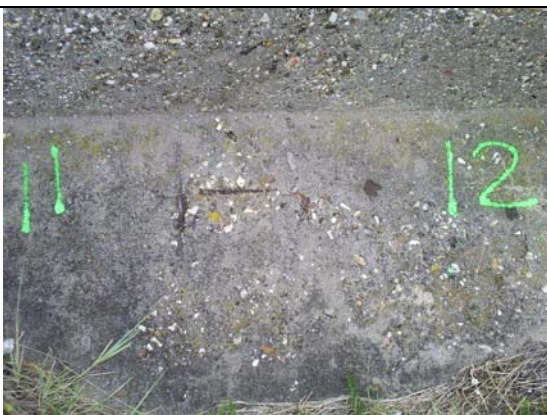
Plate 5: Schelphoek, Dijkpaal No. 55 - c.67m: Reinforcement visible on concrete slope.
