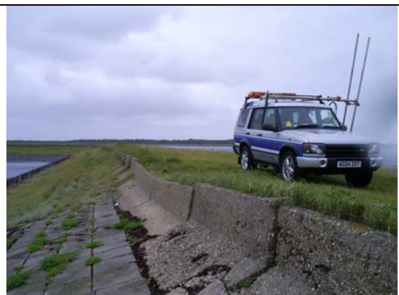
Plate 6: Schelphoek, Dijkpaal No. 55 +c.1327m Change in construction at end of dyke (near survey limit) at Schelphoek West.
