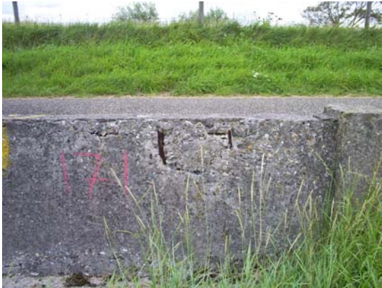
Plate 1: Viane, Dijkpaal No. 329 + c.63m: Spalling evident in wall. Reinforcement bars visible.
