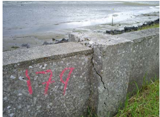
Plate 4: Viane, Dijkpaal No. 329 + 36.85m: Cracking in post.
