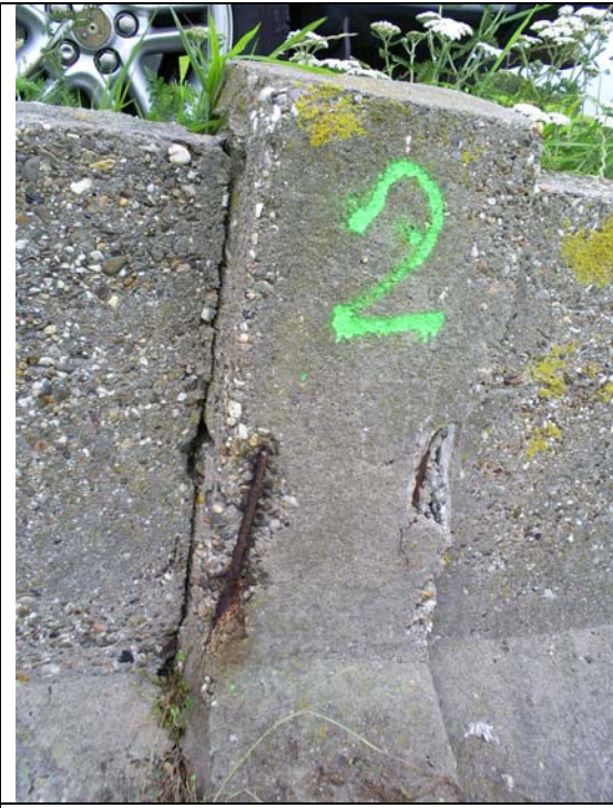
Plate 7: Schelphoek, Dijkpaal No. 55 – c.90m: Reinforcement visible on post.
