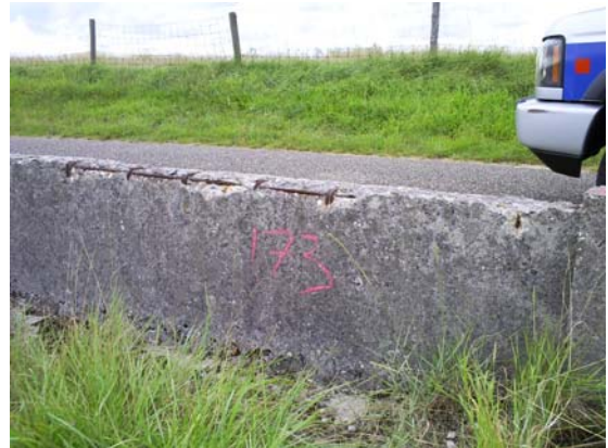
Plate 2: Viane, Dijkpaal No. 329 + c.55.5m: Reinforcement bars visible along top of wall.
