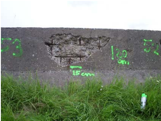
Plate 3: Viane, Dijkpaal No. 333 + c.54m: Large area of spalling in wall. Reinforcement visible. Approximate dimensions marked on wall.
